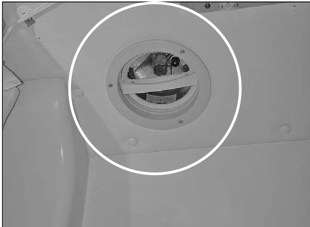
Picture B-P20: Bathroom exhaust vent.
