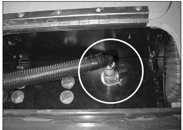
Picture G-P6: Open position of the city fresh water tank fill valve.
