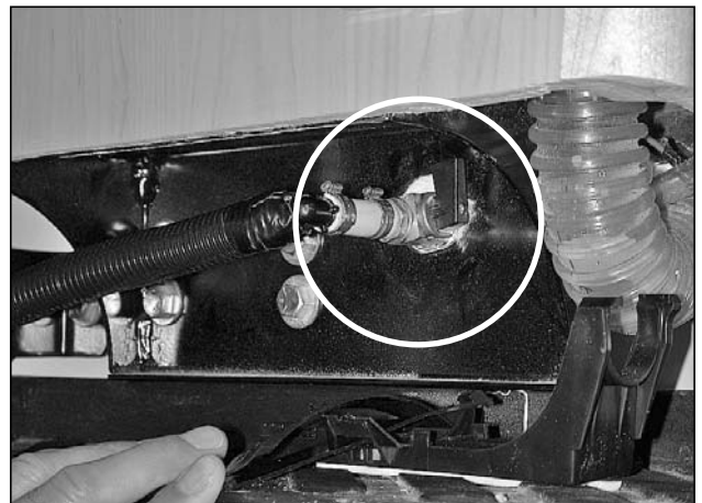
Picture G-P7: Closed position of the city fresh water tank fill valve.
