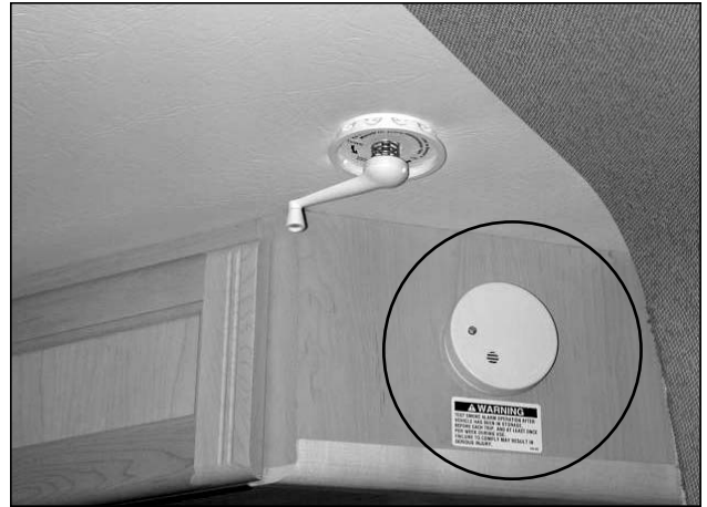
Picture F-P3: Smoke detector.
