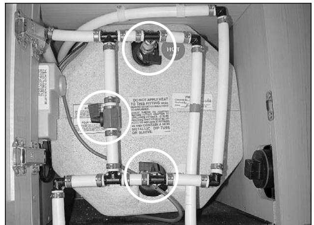
Picture G-P2: Water heater by-pass valve positions, (winter mode).
