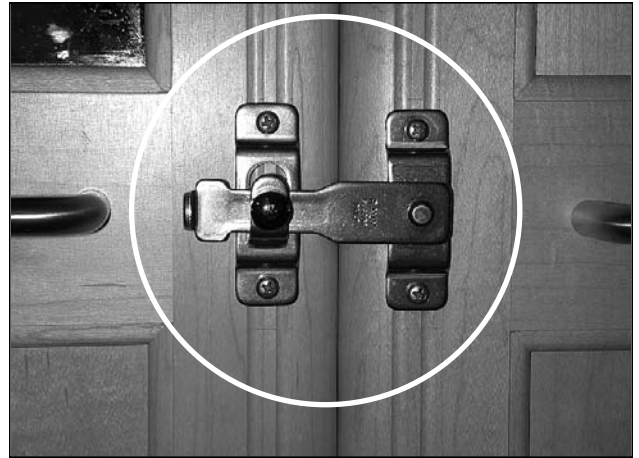
Picture B-P18: Washroom, (in transit) door latch.
